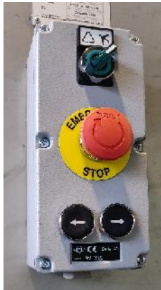
Water recirculating selector switch
